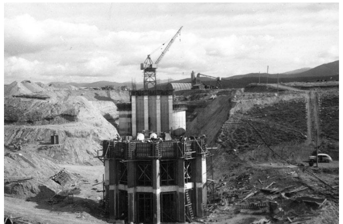
Crews construct the inlet structure to the Granby Pump Plant, later renamed to Farr Pump Plant, in September 1948.
